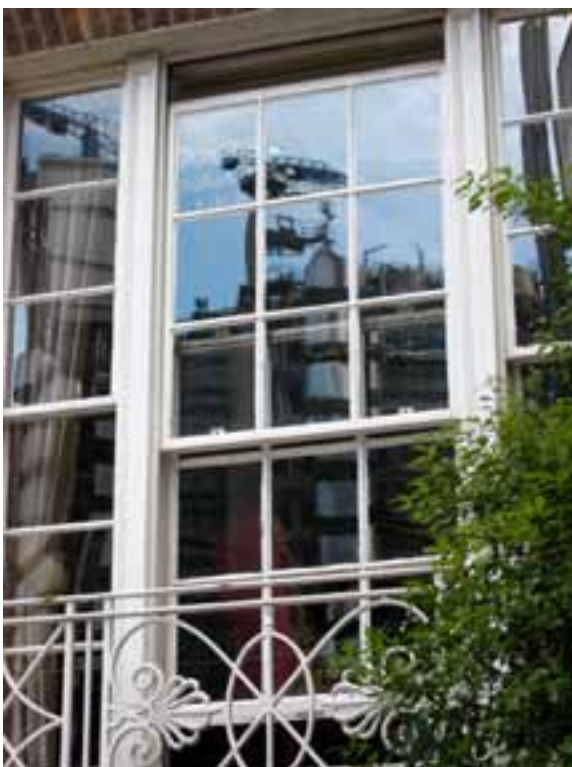
01 Historic glass should be retained in any programme of repair © Clive Murgatroyd
