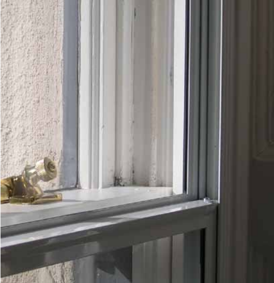
|| Secondary glazing can provide very effective draught-proofing as well as improved thermal efficiency © English Heritage/David Pickles
