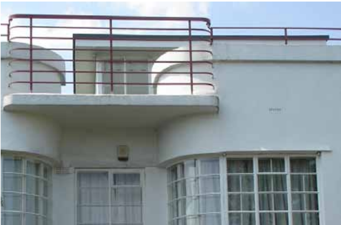
04 Metal windows can suffer from surface rust, distortion and excessive build up of paint but they are capable of repair. © English Heritage/ David Pickles
